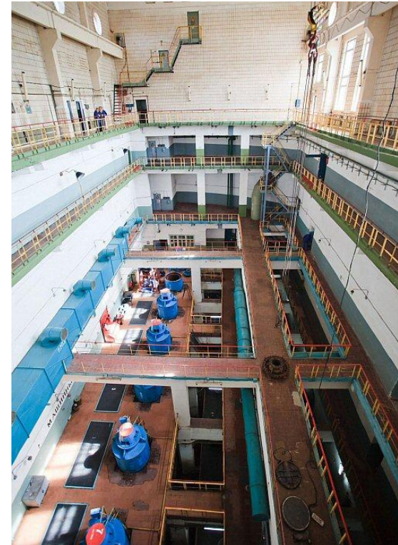
Pumping room of BSA
